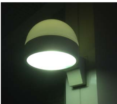
Figure 1: Large lights around atrium.
